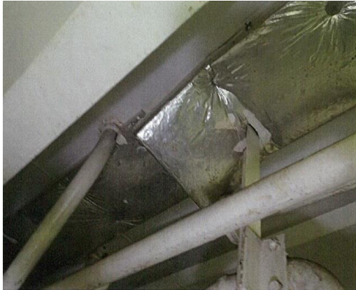
Deteriorated insulation on underside of deck.
