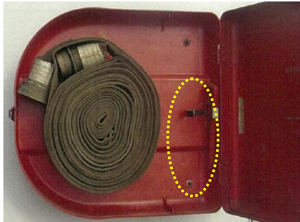
Hose nozzle missing.
