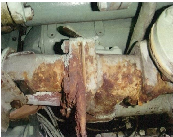
Badly corroded and leaking piping.
