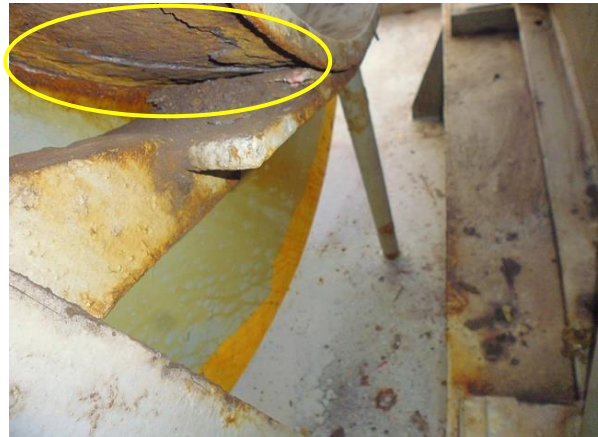
Poorly maintained windlass brake.
